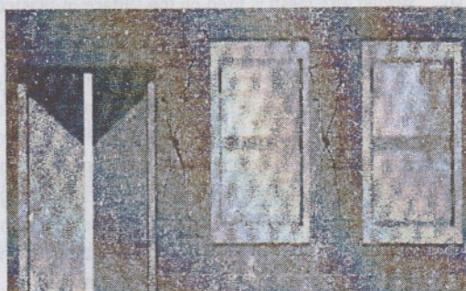
Fig. 8: Cracks between openings
