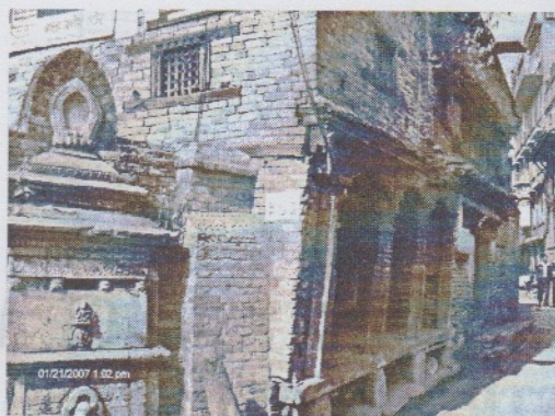
Fig.2: Damaged Brick Masonry Building
